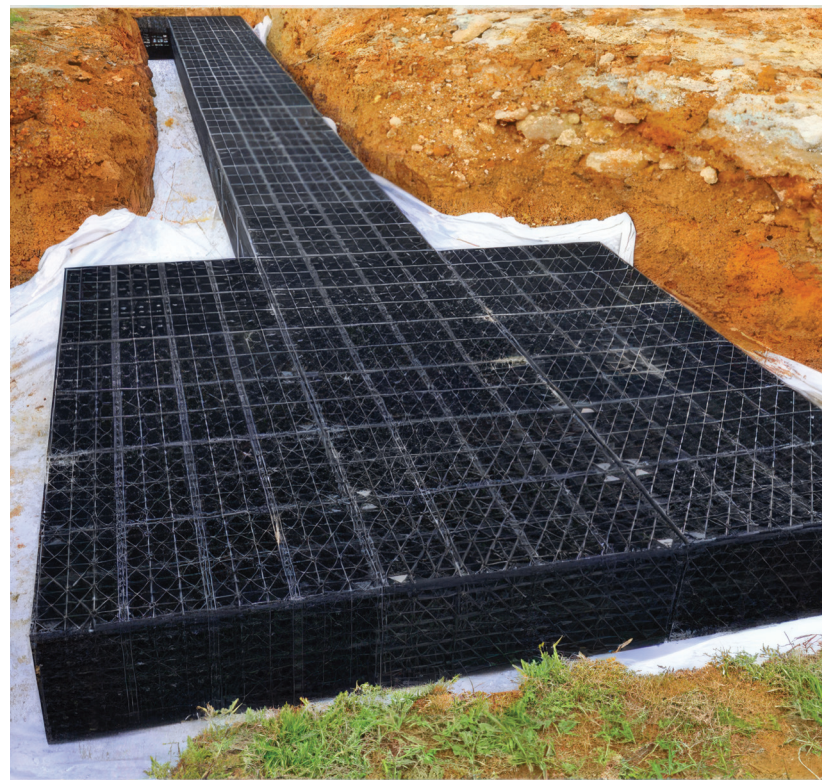
Bladder tanks to hold rain water for irrigation
