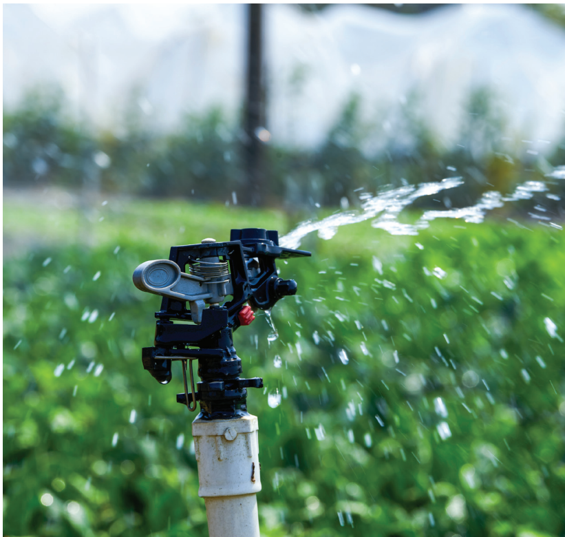
Facility for irrigation
